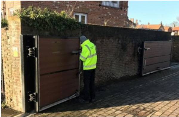
Yarm flood gates
