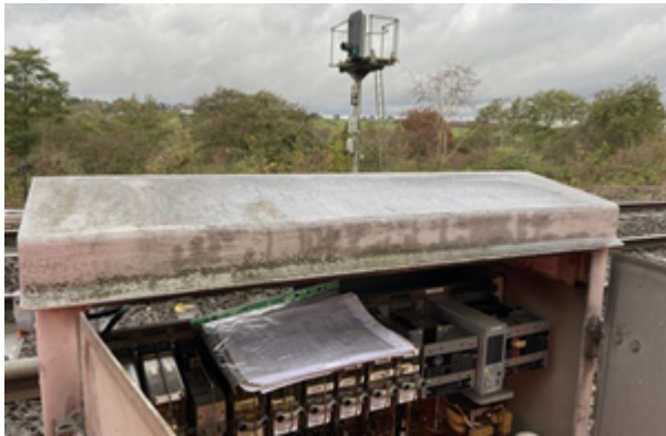
Signal DY586 and its signalling location cabinet
