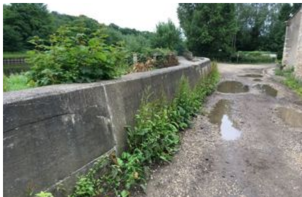
The damaged flood wall at Sprotbrough
