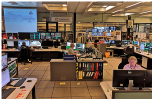
The JET control room
