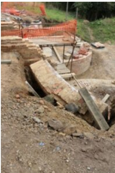
A section of the wall collapsed while Mr
