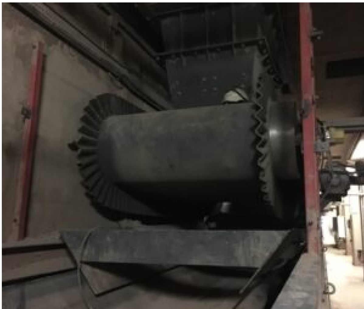
The feed hopper and conveyor at Mountsorrel Quarry
