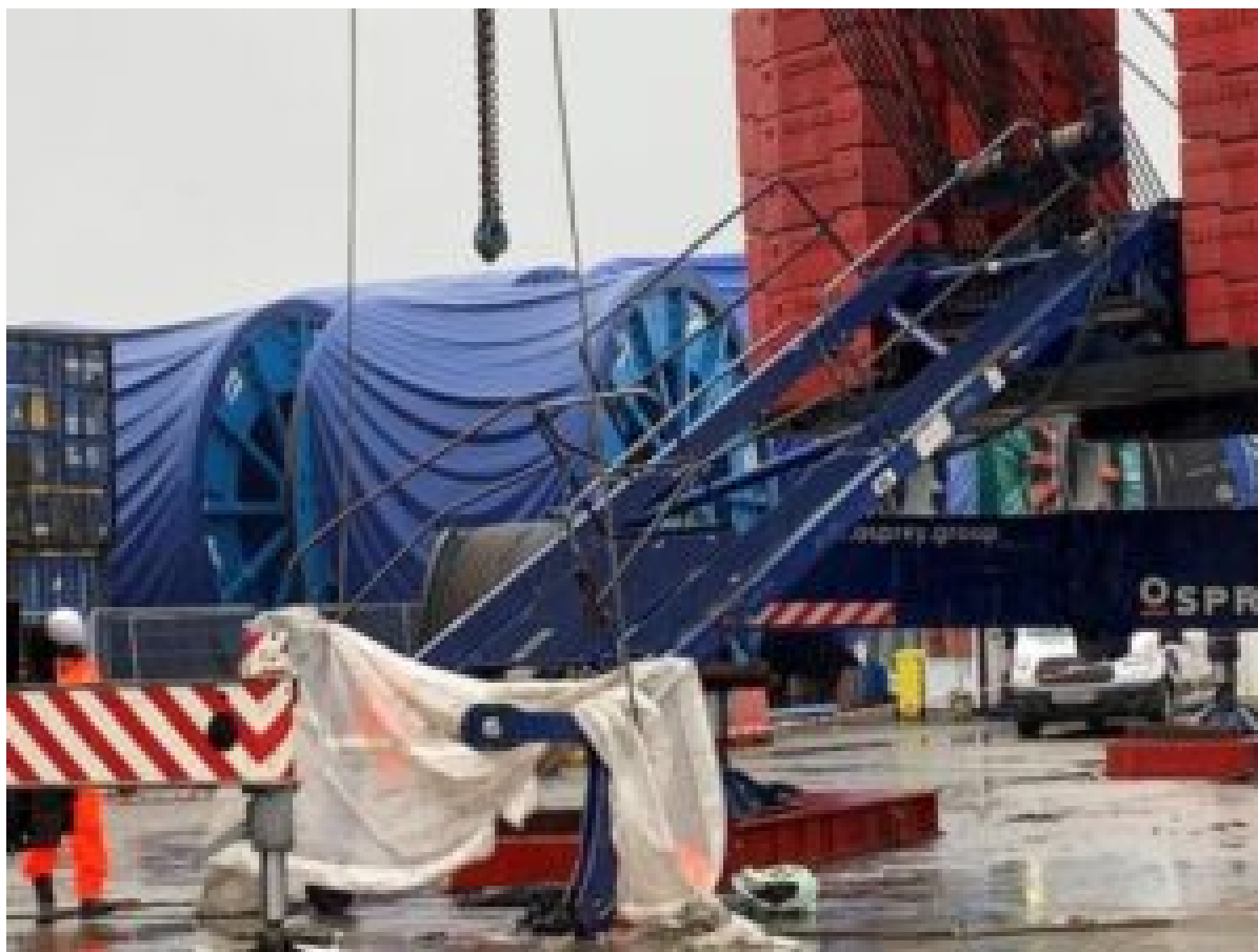
The collapsed platform
