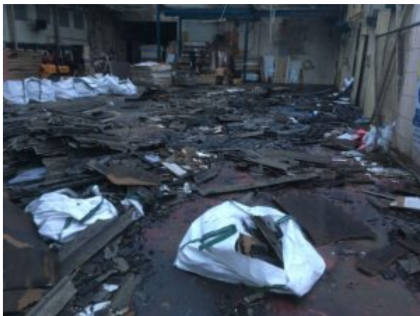
Some of the asbestos containing materials on site
