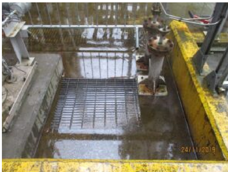
Photo of sump with grating in place taken shortly
