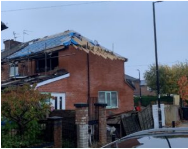
Abdul Rehman carried out unsafe work on his own house in Old Trafford
