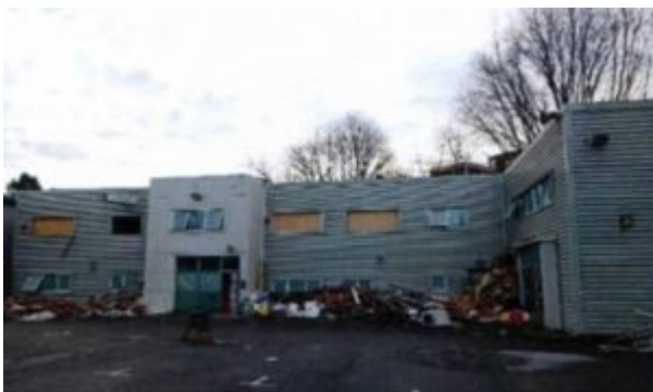
Debris outside the Cavendish centre
