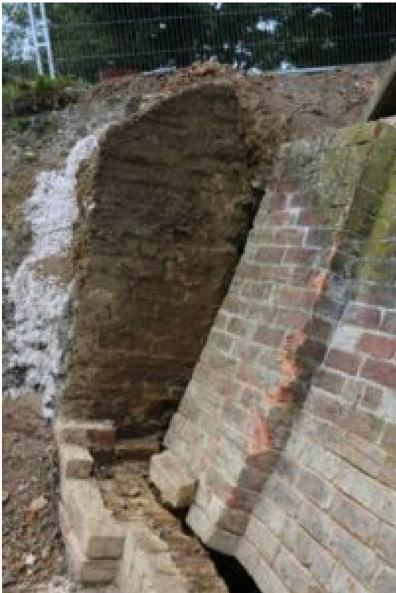
A section of the wall collapsed while Mr Konitzer was inside the excavation
