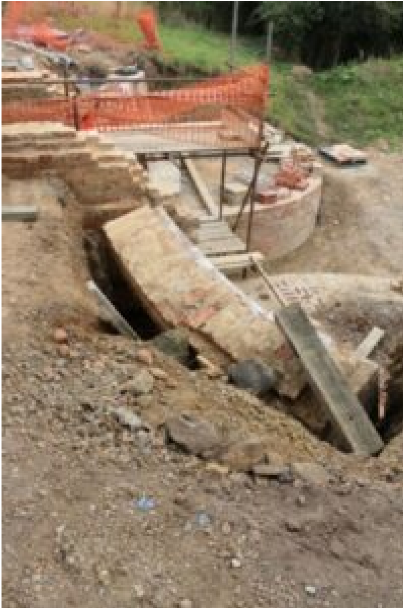
A section of the wall collapsed while Mr Konitzer was inside the excavation
