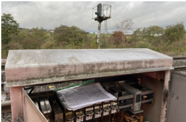
Signal DY586 and its signalling location cabinet
