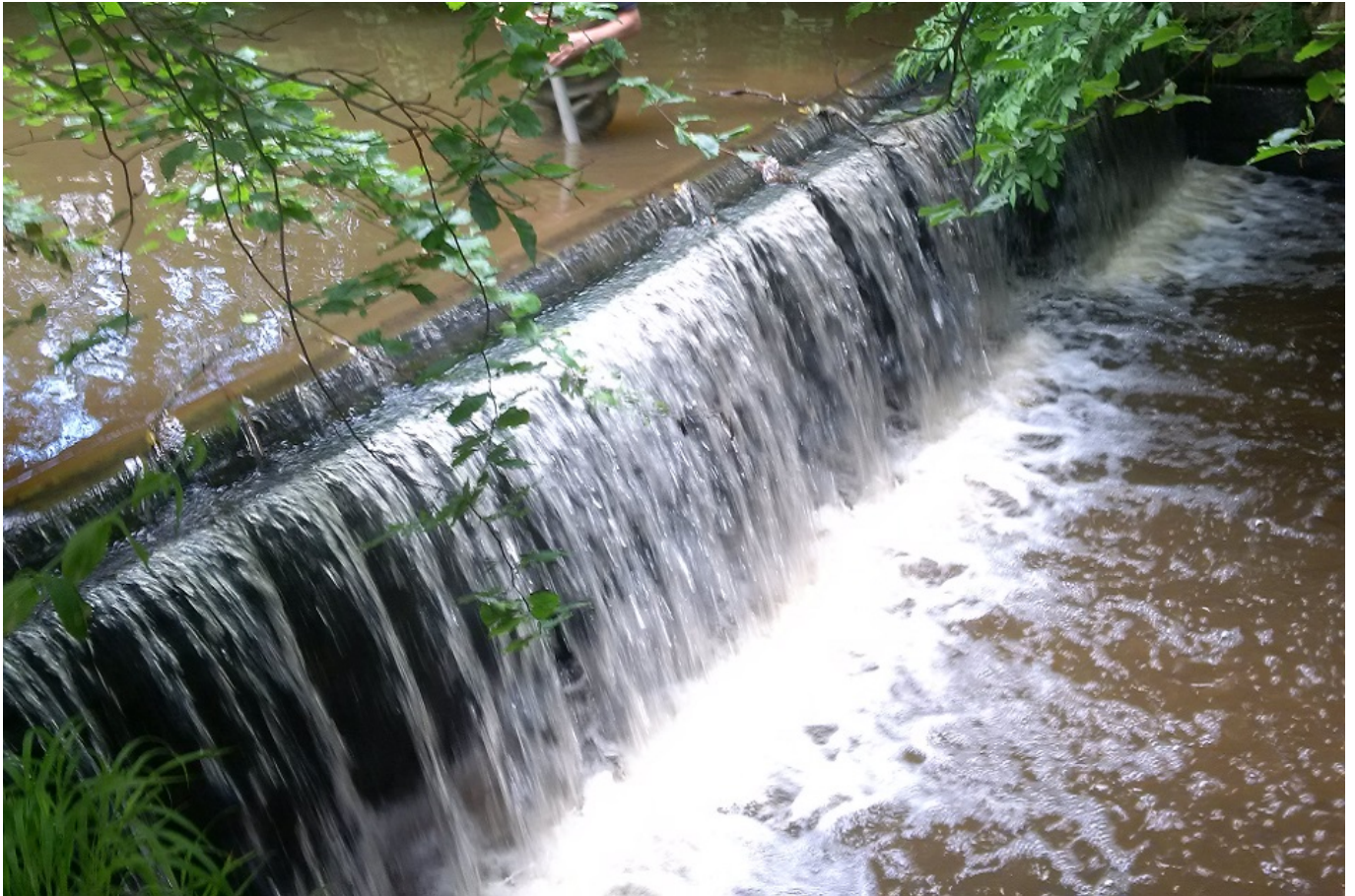
Upstream weir before it was altered to make it easier for fish migration
