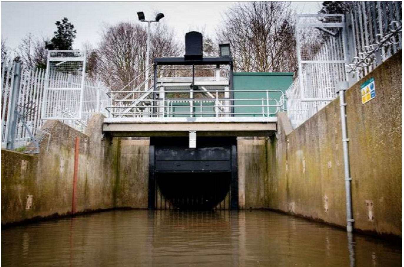
The lifting screen at Primrose Hill
