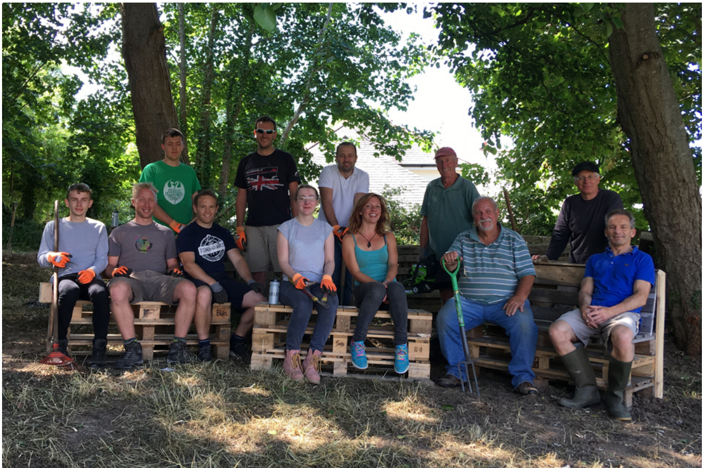
The Highways England team, including assistant project manager Karl Sullivan fourth left, and Chacewater villagers, with Rob Knill third from right, and the team busy clearing vegetation
