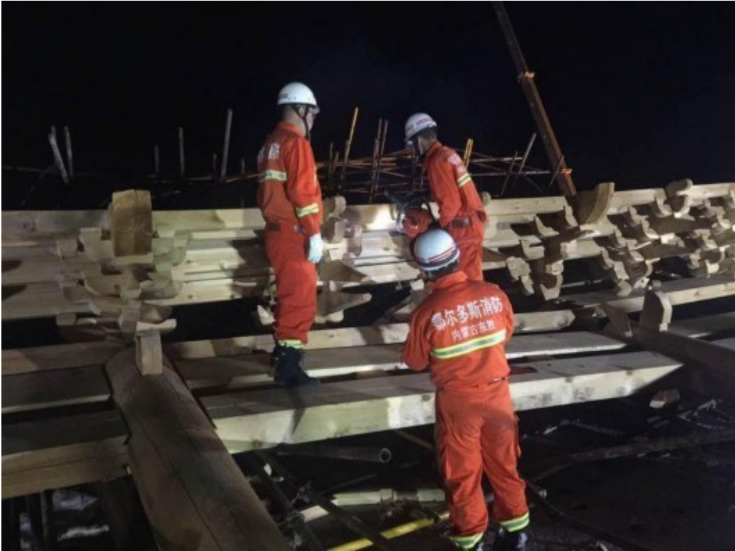
Rescuers work at the scene after a construction site collapse in Inner Mongolia. [Photo/Shanghai Daily]
