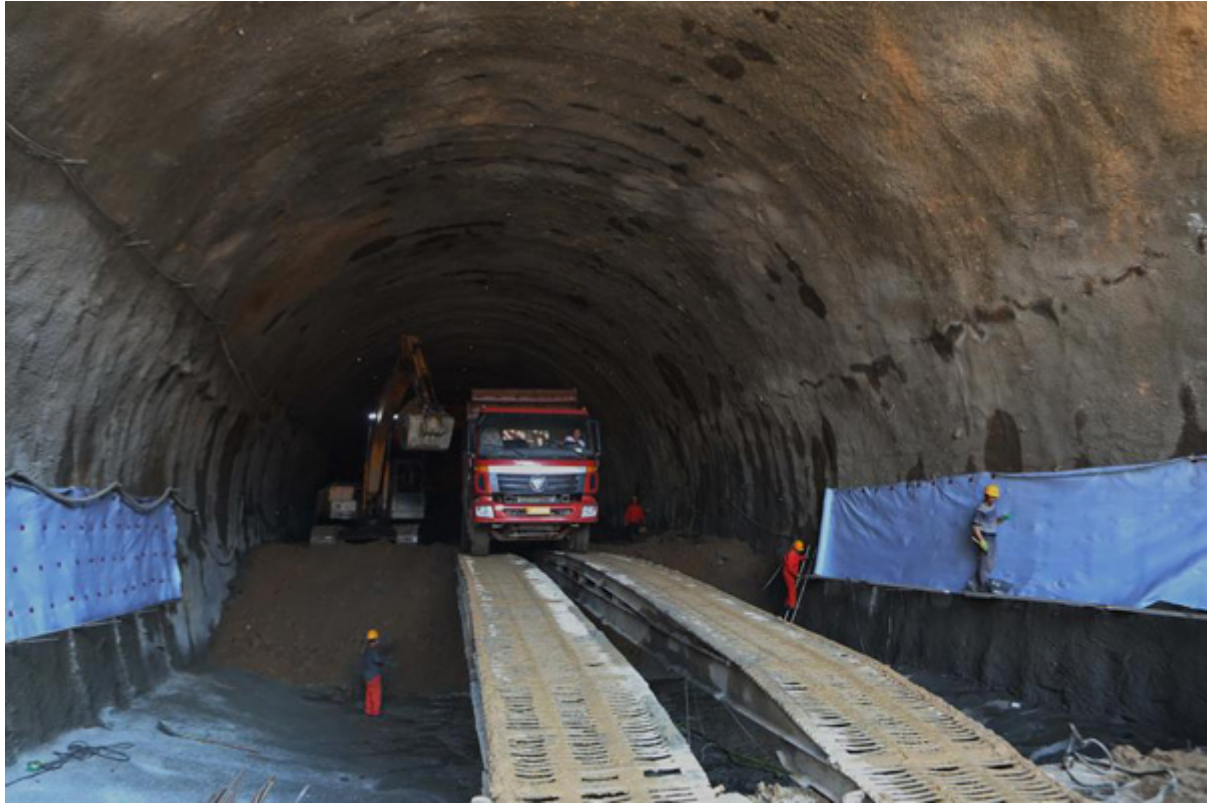
Workers are digging a tunnel of the Beijing-Zhangjiakou high-speed railway line's branch linking Chongli county, Zhangjiakou, Hebei Province, on June 30, 2017. [Photo/Xinhua]
