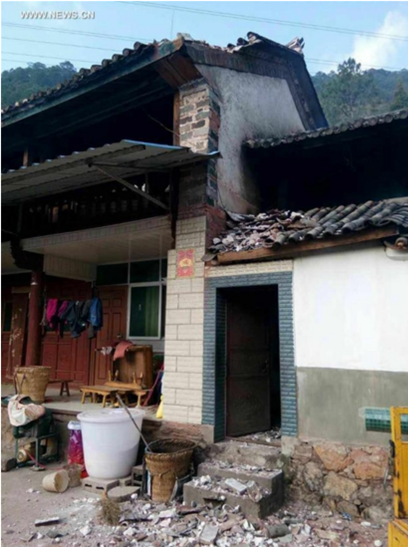
Photo taken on March 27, 2017 shows damaged houses at quake-hit Puping Village of Yangbi County in southwest China's Yunnan Province. [Photo/Xinhua]
