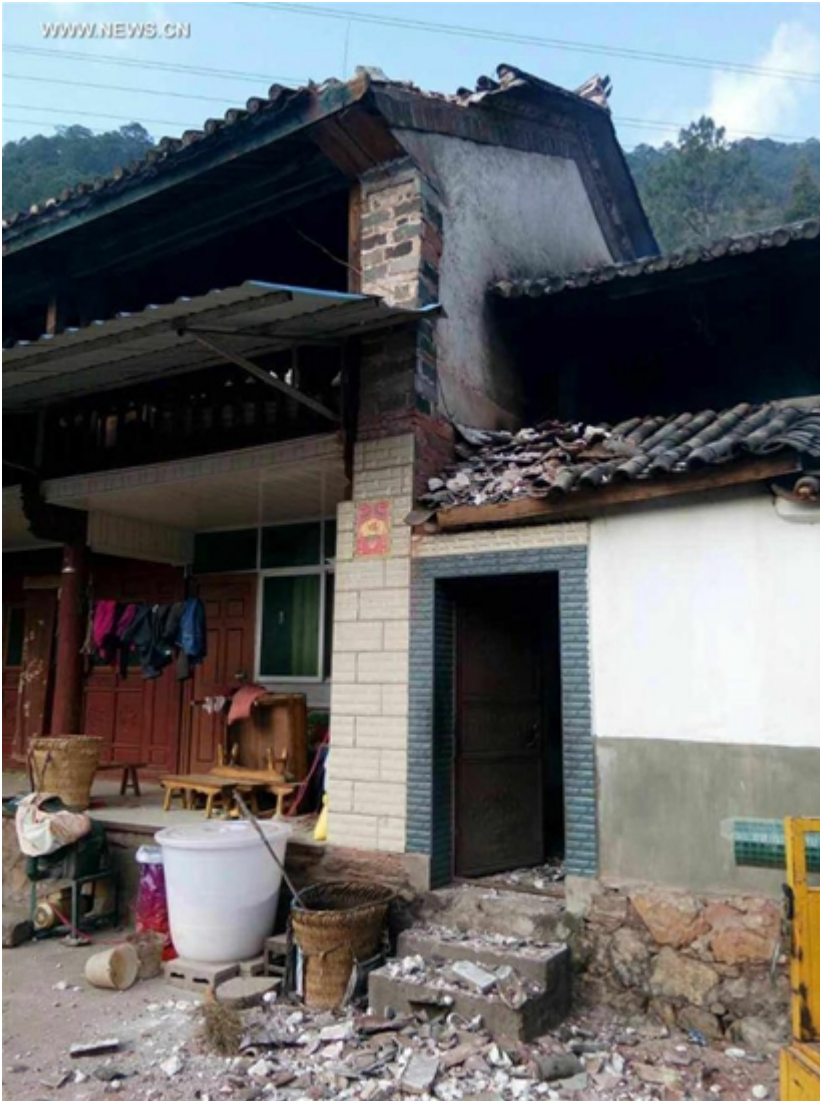
Photo taken on March 27, 2017 shows damaged houses at quake-hit Puping Village of Yangbi County in southwest China's Yunnan Province. [Photo/Xinhua]
