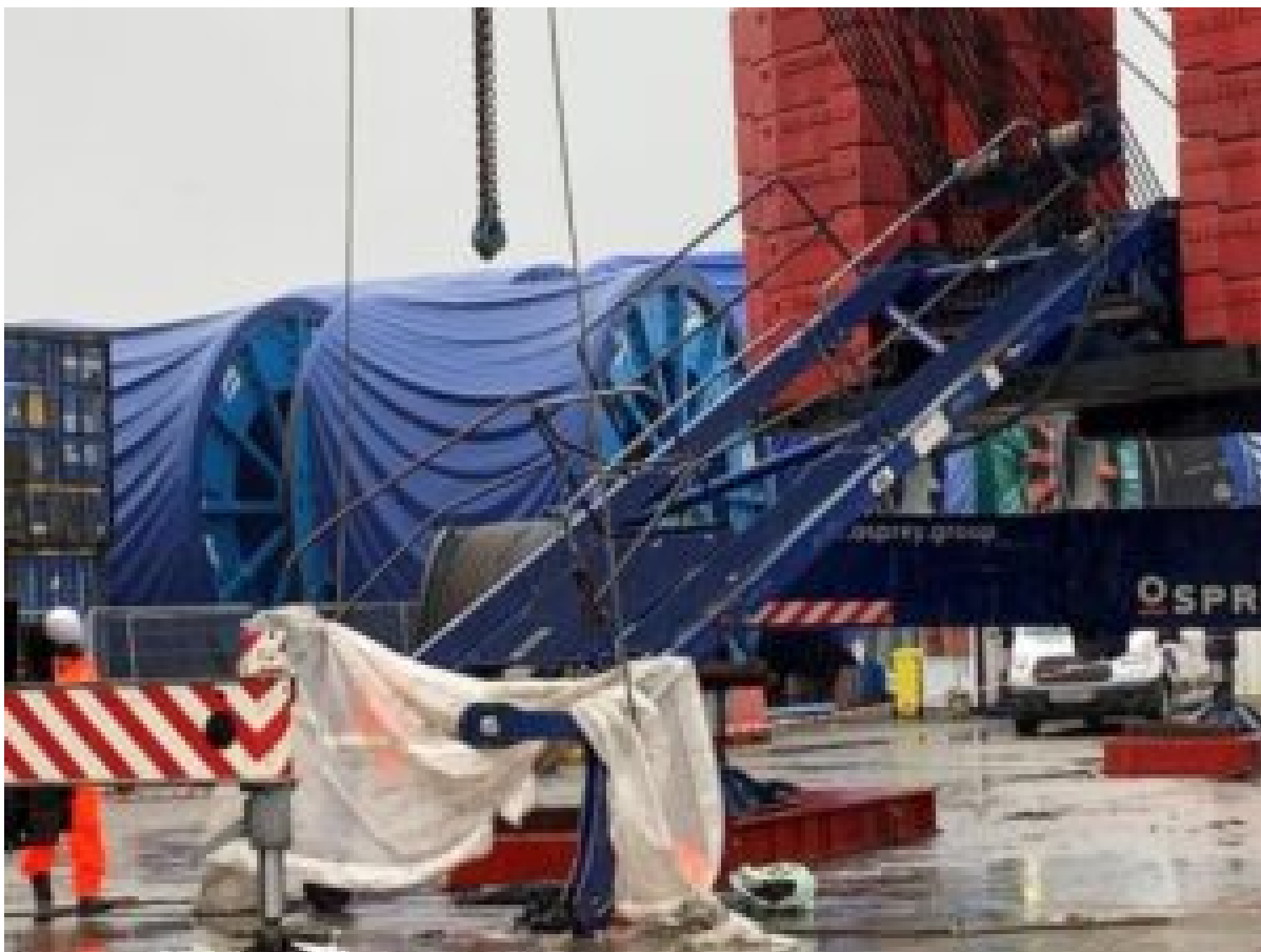
The collapsed platform
