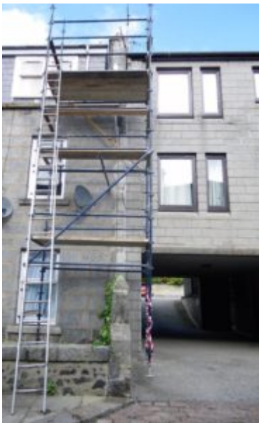
Unsafe scaffold at Jute Street
