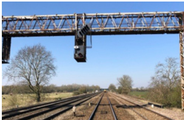
Signal LR507 (image courtesy of Network Rail)
