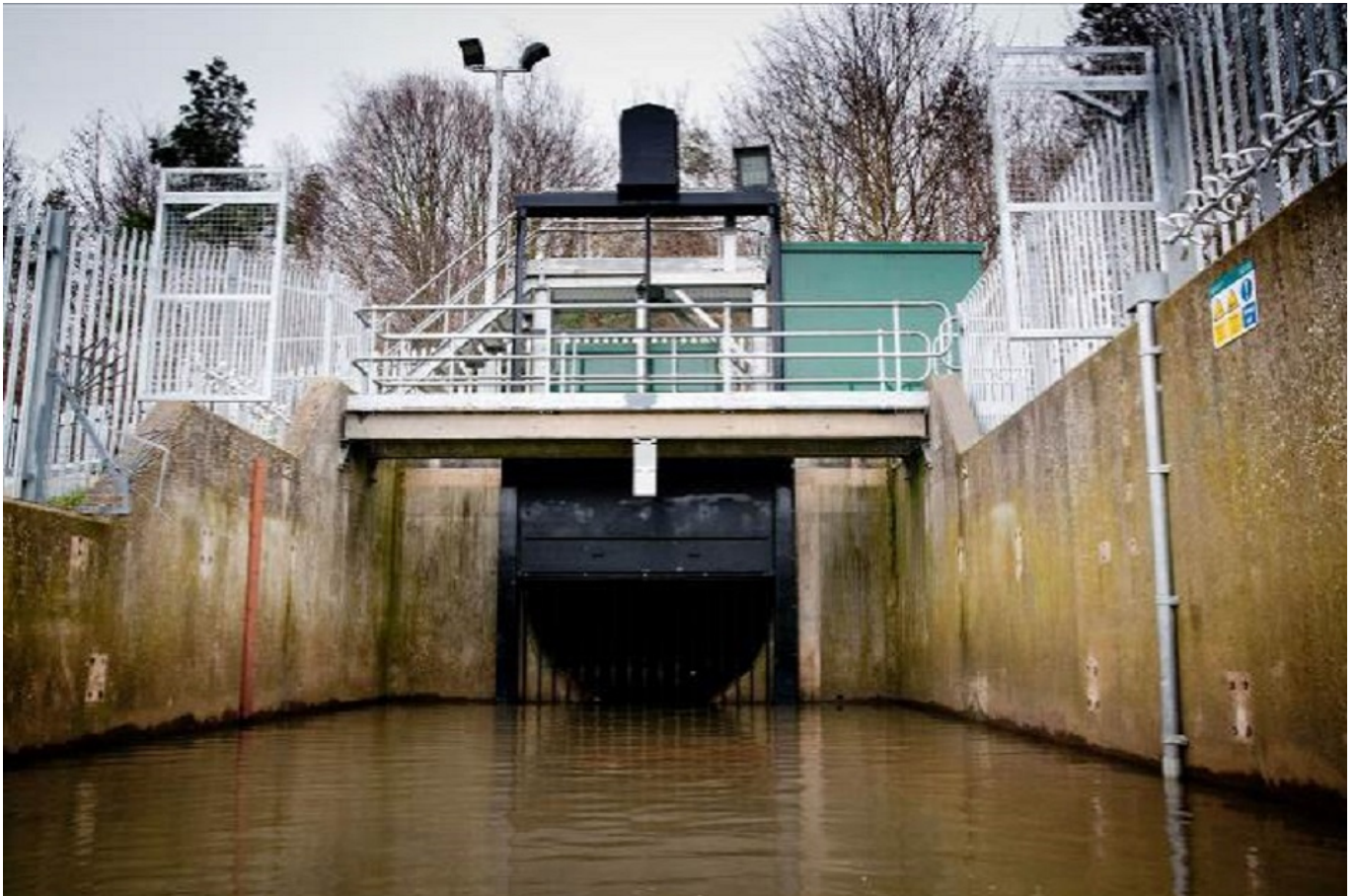
The lifting screen at Primrose Hill
