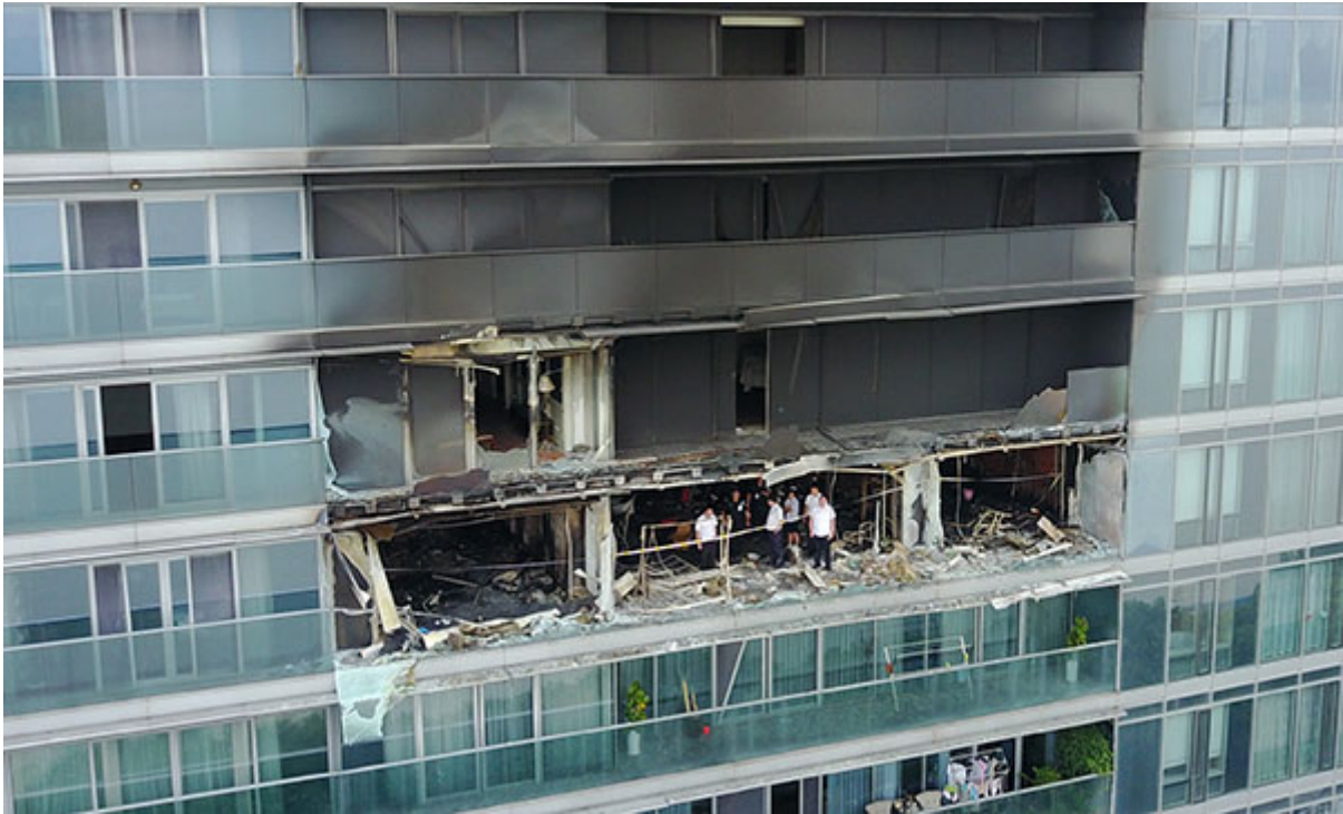
The apartment after the fire.[Dong Xuming/For China Daily]
