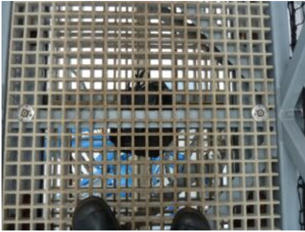
Mr Hill's trapped boot in the gangway
