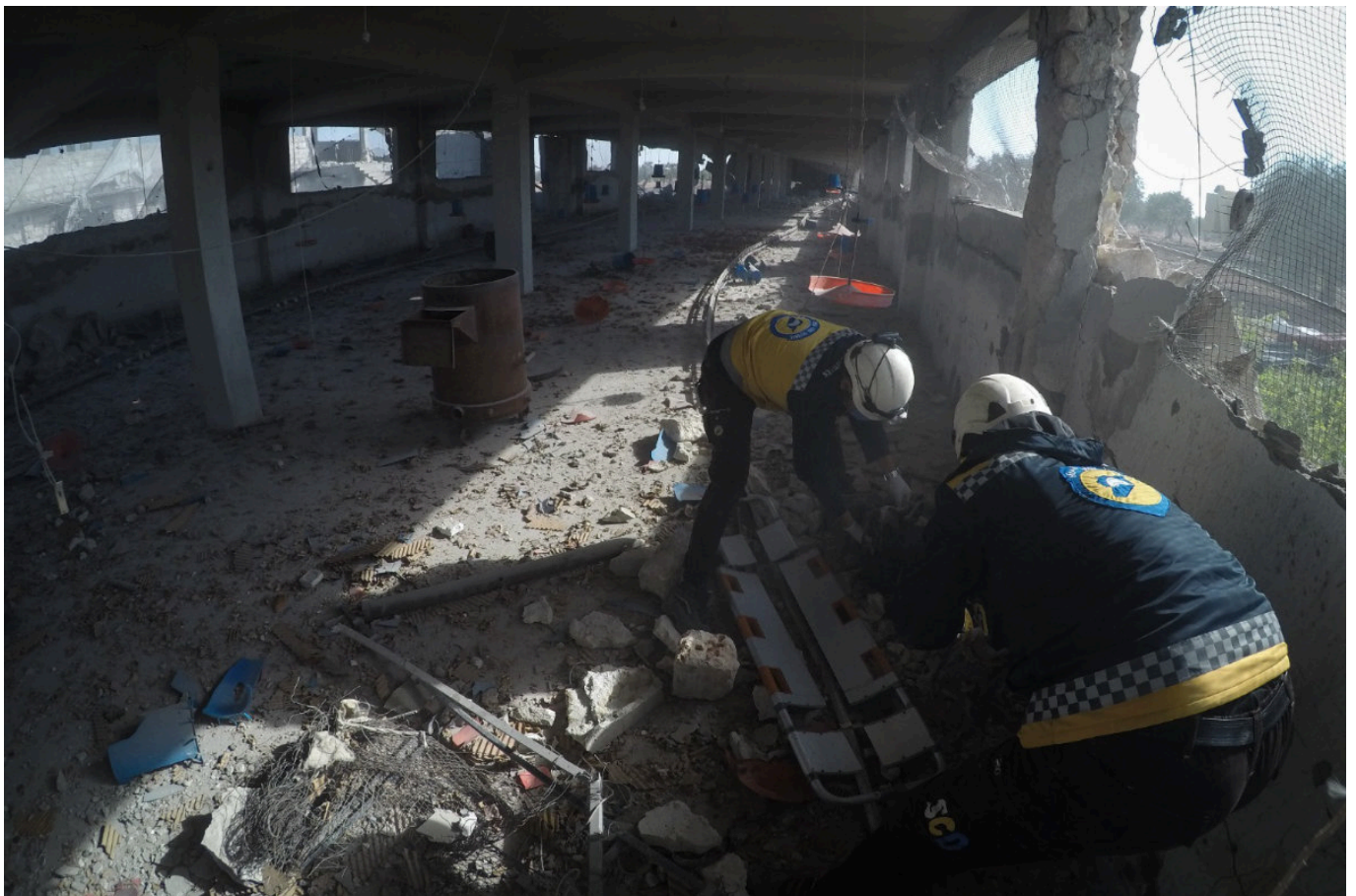
Syria's White Helmets volunteers search through the rubble of a building destroyed by an exploding bomb in Idlib. (AFP file photo)
