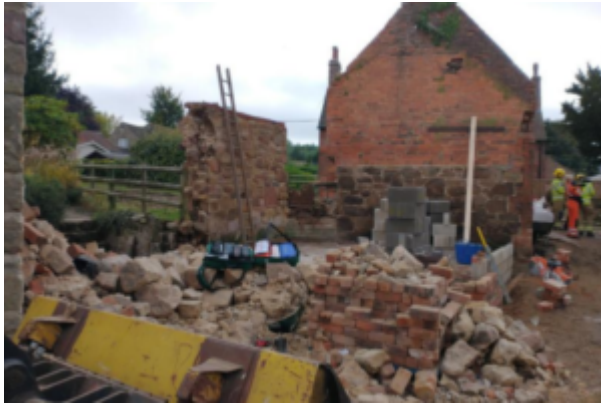
The site where the wall collapsed in Woodhouses, Derbyshire
