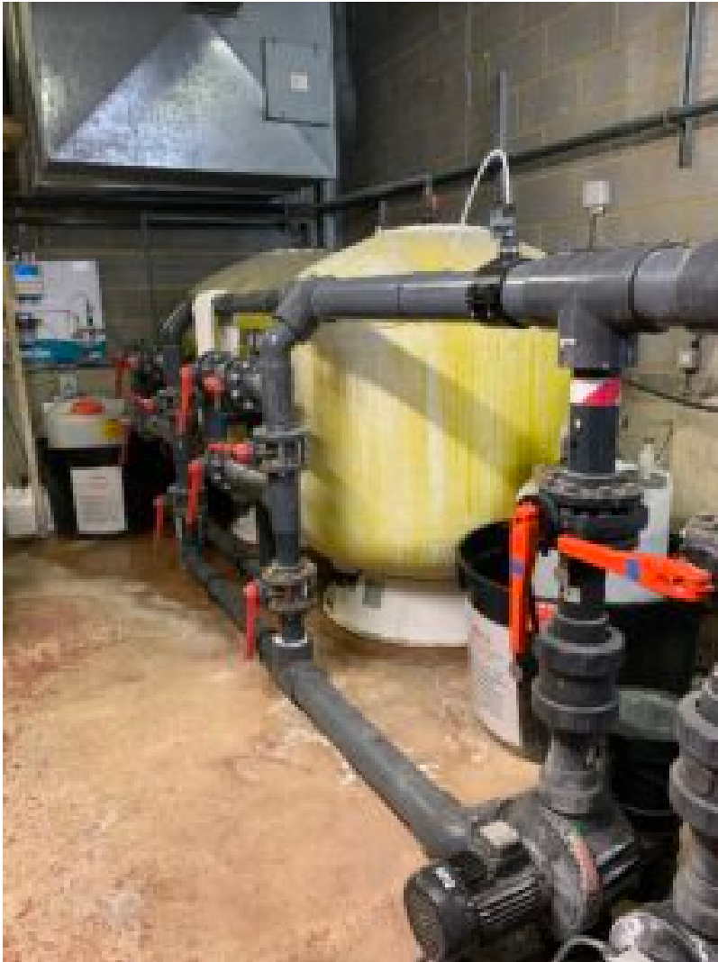
The sodium hypochlorite tank at The Hampshire Clinic
