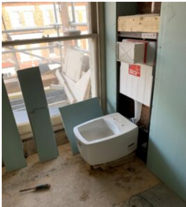
The unusable toilet on site
