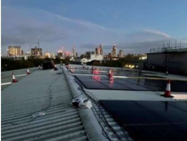
Cones used to mark out location of fragile skylights
