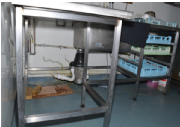
Bishops Wood Hospital kitchen area – sink and macerator underneath
