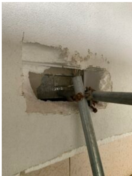
Combustible material exposed where scaffold is attached to the building
