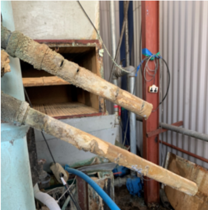
One of the water-cooling towers at Riaar Plastics Limited
