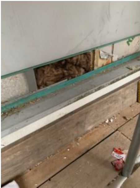
Exposed combustible material on exterior of the building
