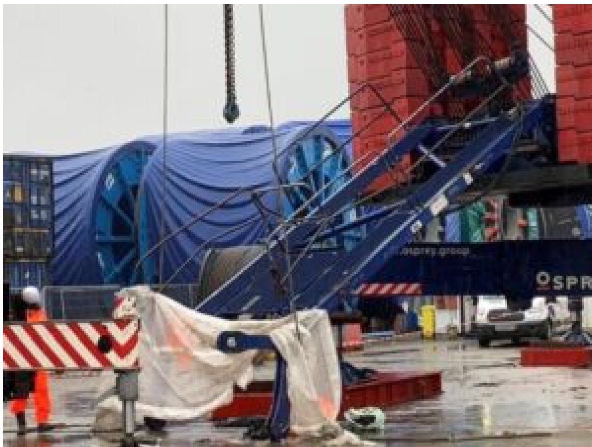
The collapsed platform
