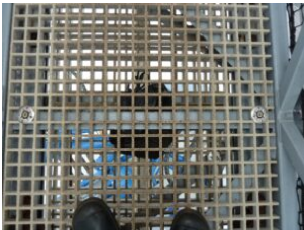
Mr Hill's trapped boot in the gangway
