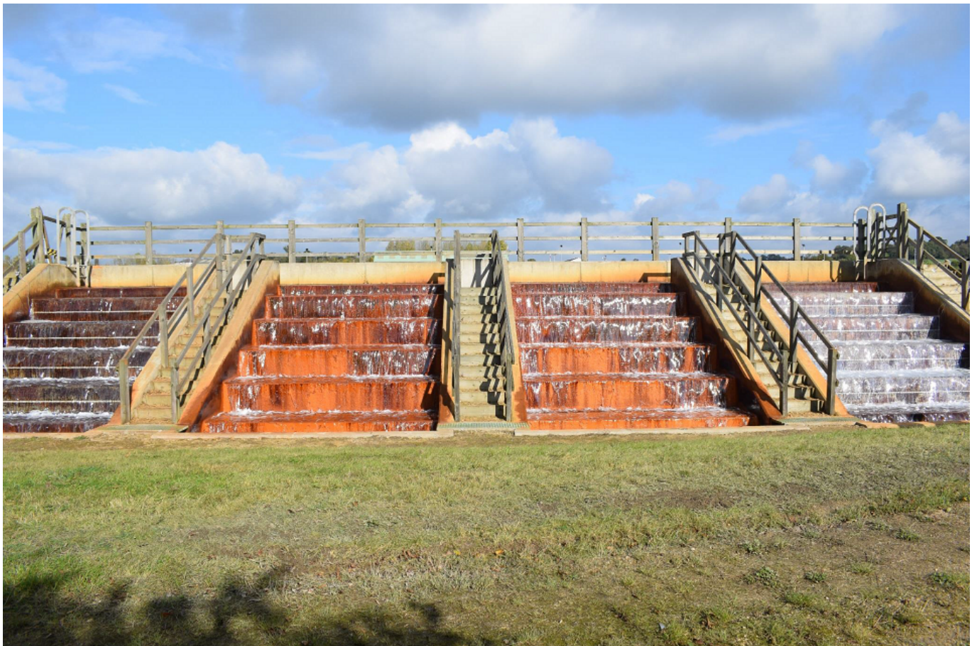
The 4 water cascades at the mine water treatment scheme
