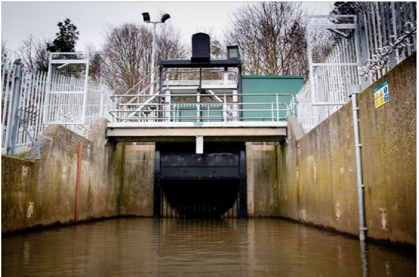
The lifting screen at Primrose Hill
