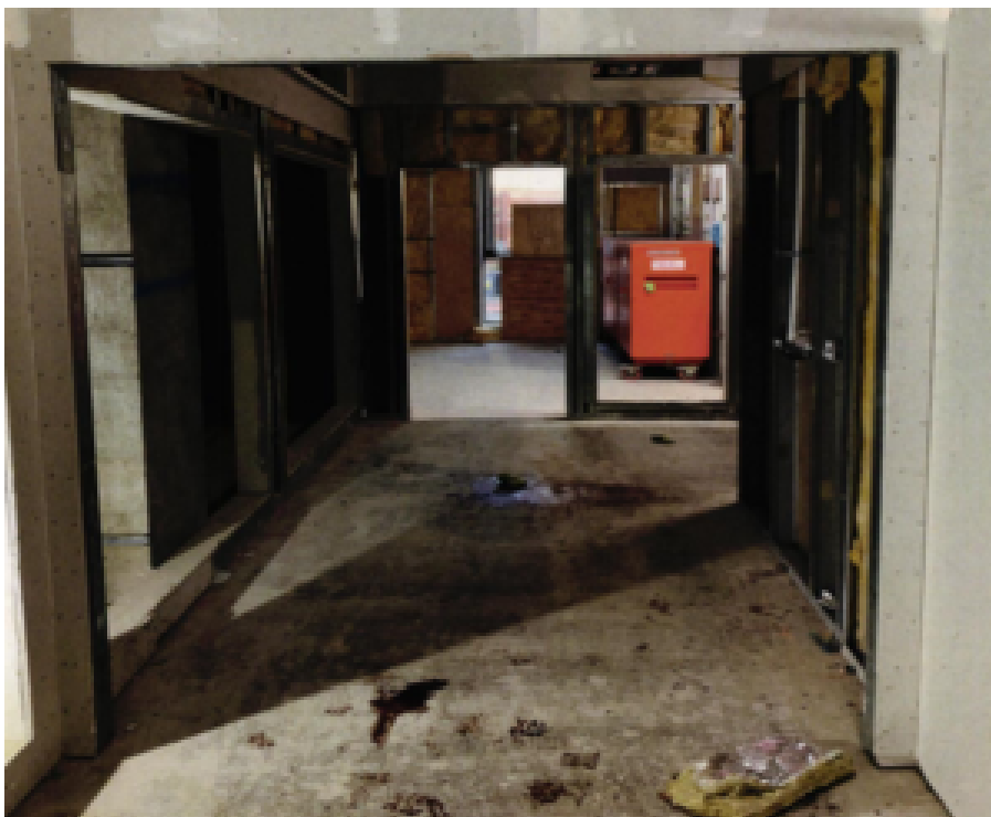
Area of the corridor where the incident occurred
