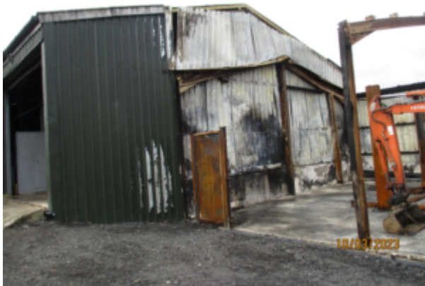
The barn which roof the man fell through
