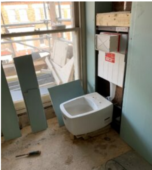
The unusable toilet on site
