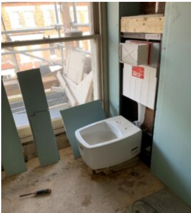
The unusable toilet on site
