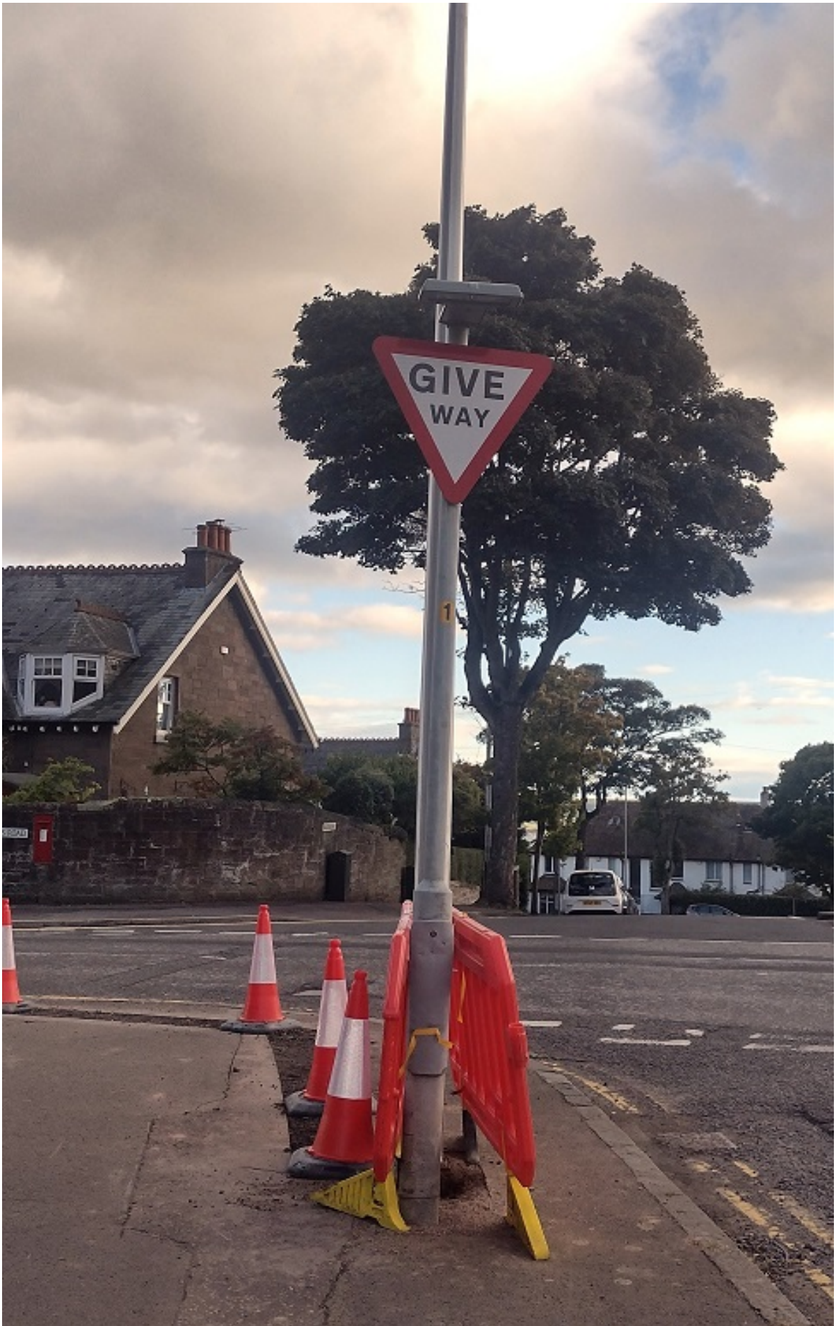
Further to our August update on planned road safety improvements at the
