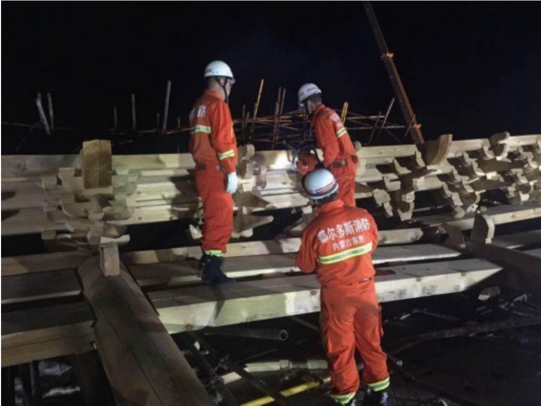
Rescuers work at the scene after a construction site collapse in Inner Mongolia. [Photo/Shanghai Daily]
