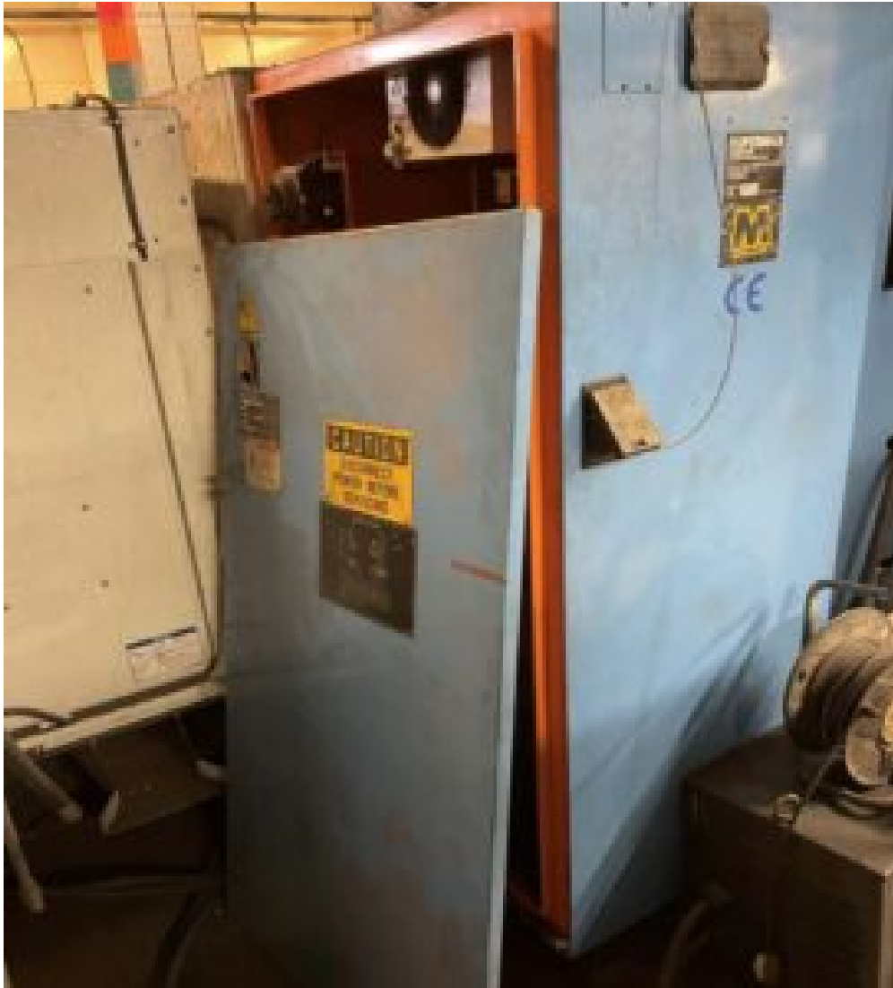
High voltage panel removed while machine in operation
