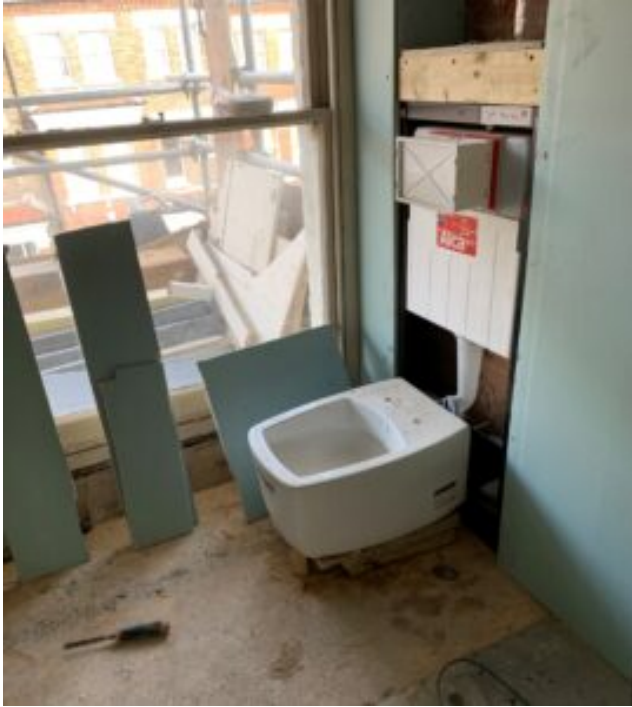
The unusable toilet on site
