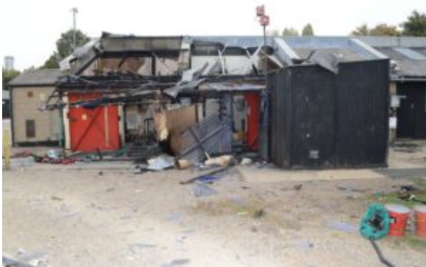
The aftermath of the explosion at Le Maitre Limited
