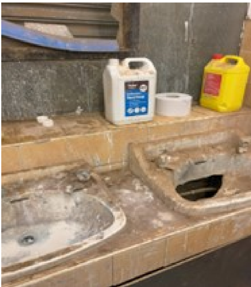
Some of the company's local exhaust ventilation (LEV) systems, which are used
