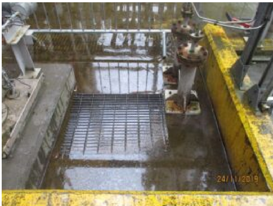
Photo of sump with grating in place taken shortly after the incident
