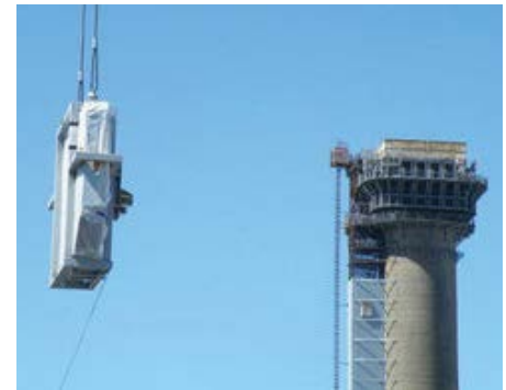
Once each hole is cut in the silo, the section of concrete is cut away in a single piece (known as a monolith)
