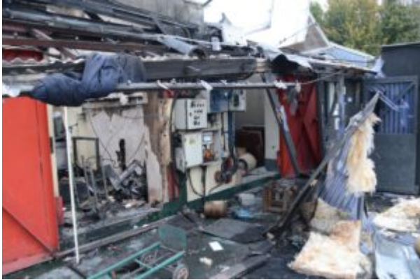
The aftermath of the explosion at Le Maitre Limited
